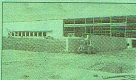
The south side of the exterior of the beef plant under construction south of Aberdeen.
